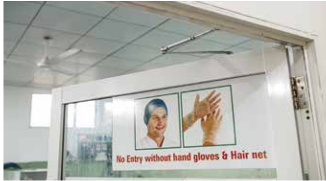
Photo 7: Door with self-closing hinge and non-absorbent surface
