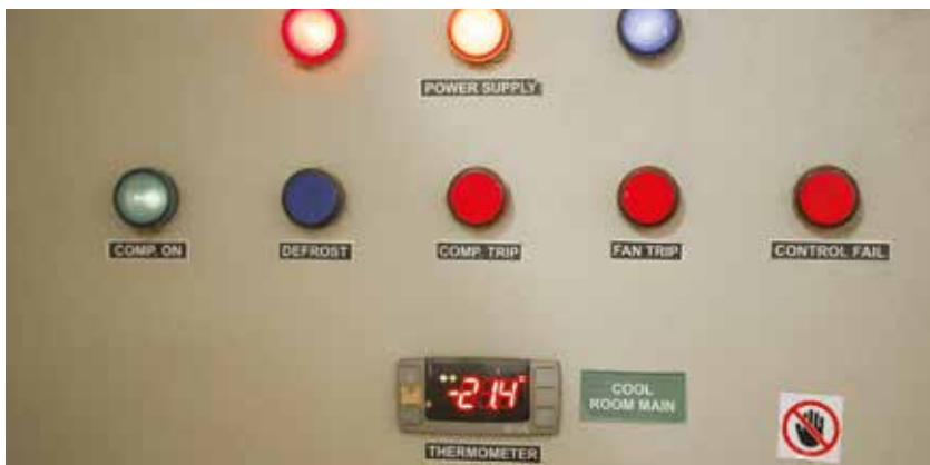
Photo 21: Control panel of a cold room with temperature indicator
