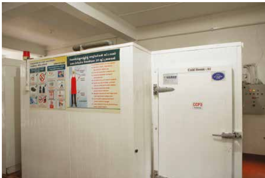
Photo 18: Cold store of an ice-cream factory
