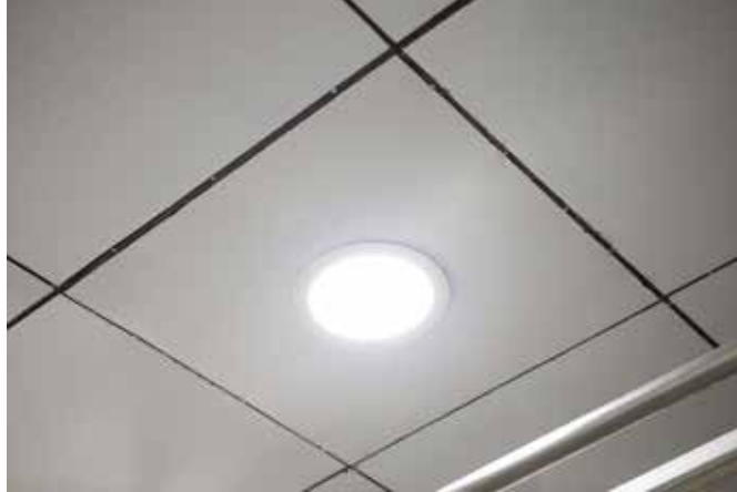
Photo 11: Lighting with a covered bulb
