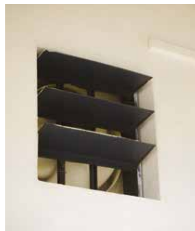
Photo 10: Ventilation with screens
