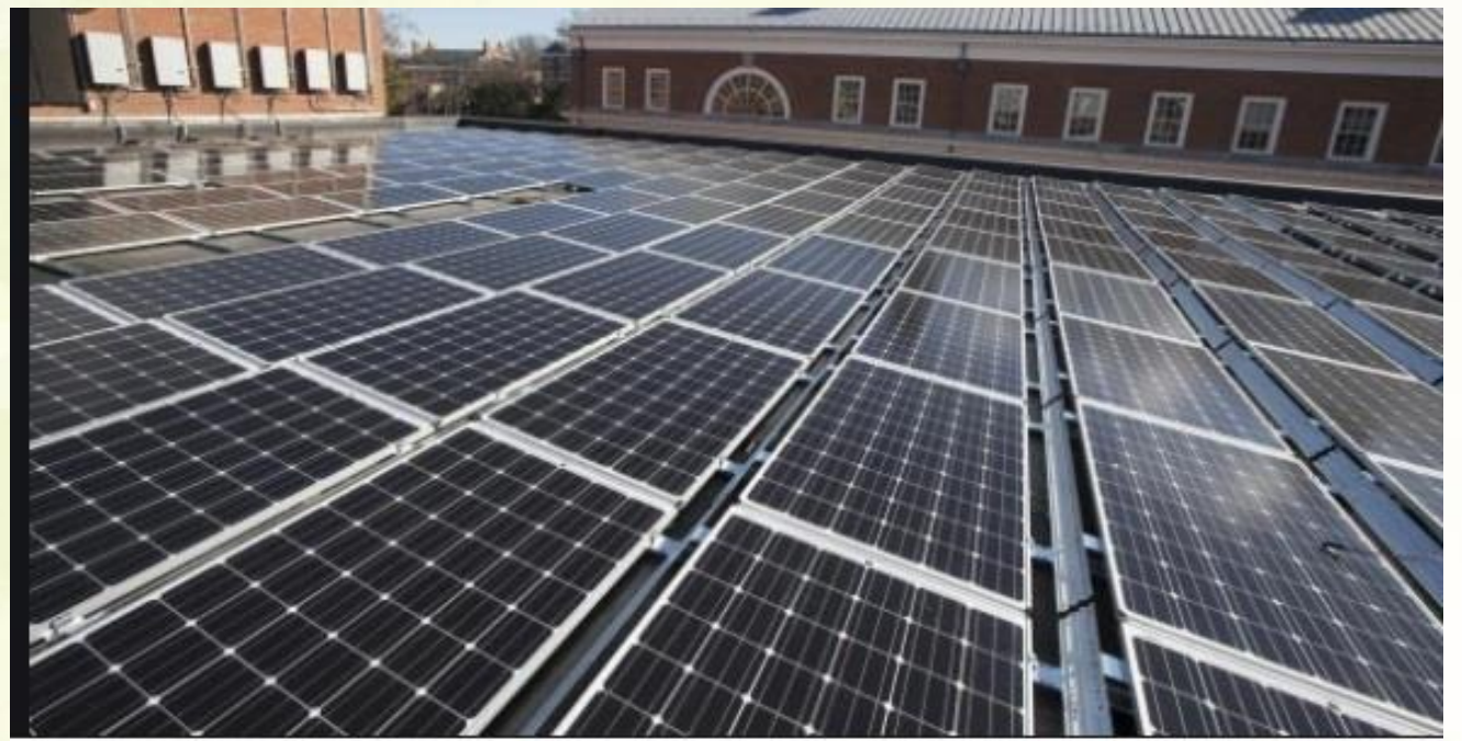
SOLAR PANELS ON ROOF TOPS
