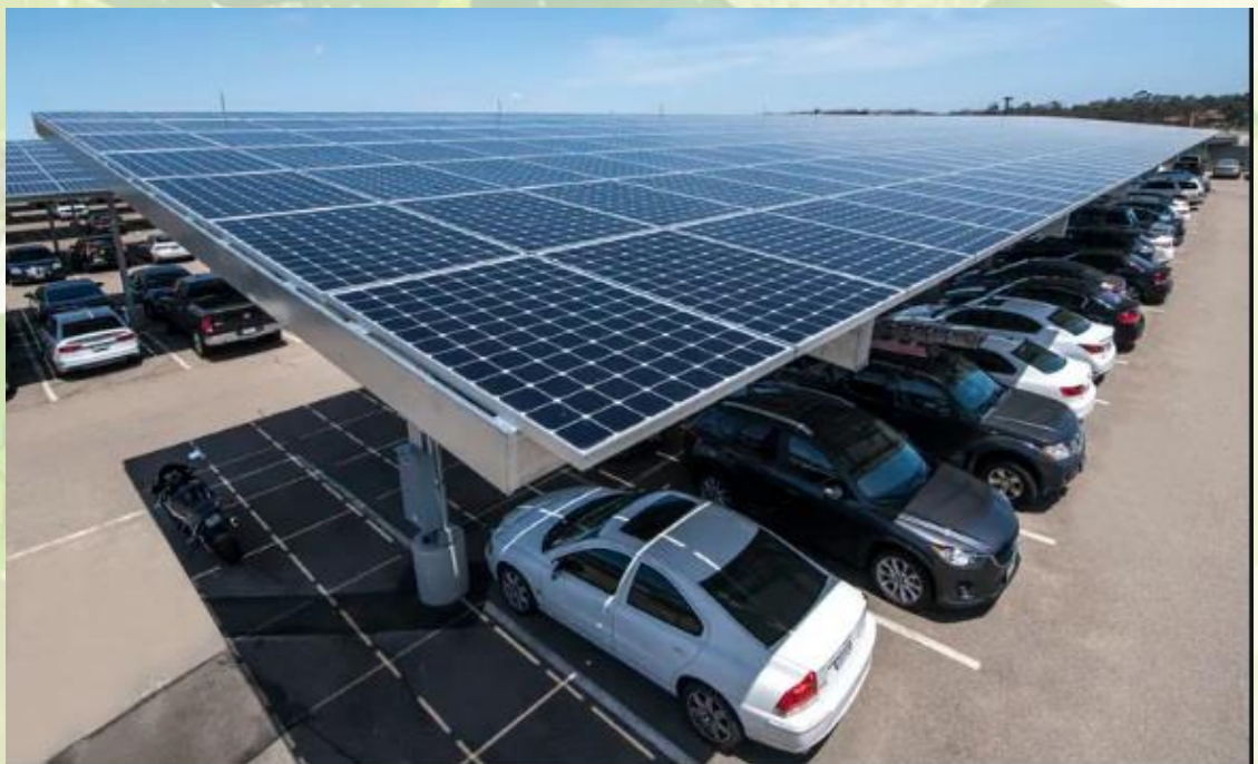
SOLAR PANEL SHADED CAR PARKING PLOTS
